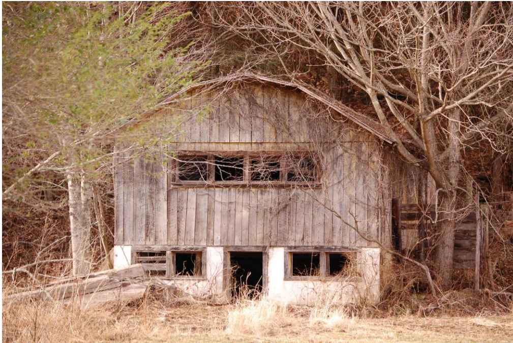
Figure 7: Apple House at the Lee Little Barn and Outbuildings, south elevation, view to north-northeast
