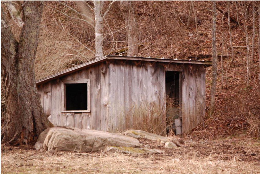
Figure 8: Chicken House at Lee Little Barn and Outbuildings, south elevation, view to north-northwest
